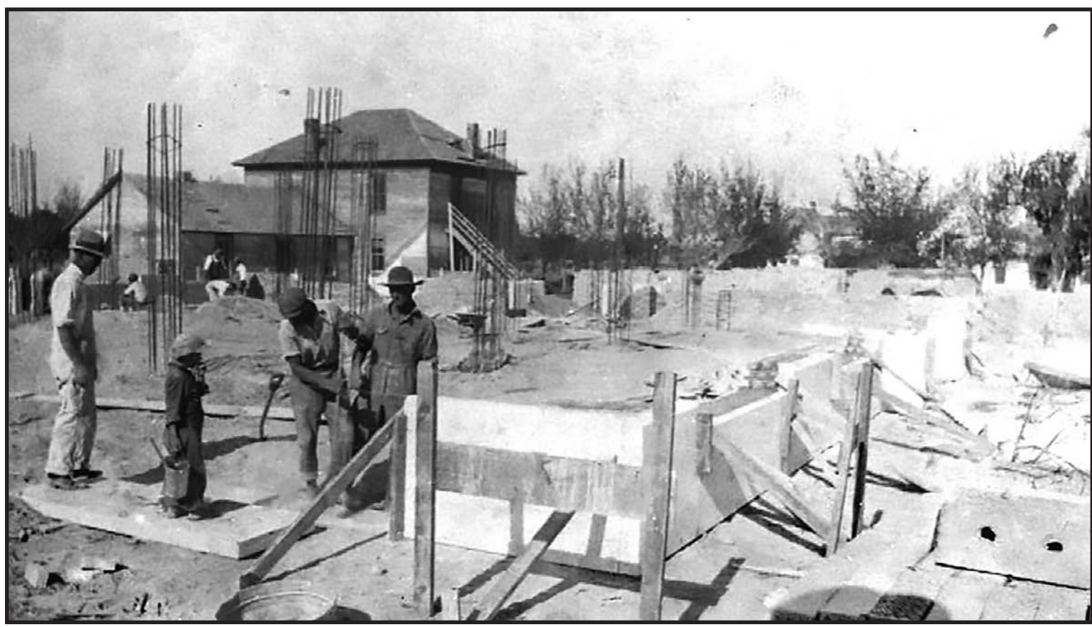
Starting on the foundation of the new Courthouse, 1917. (Photo courtesy of Sheridan County Historical Society)
